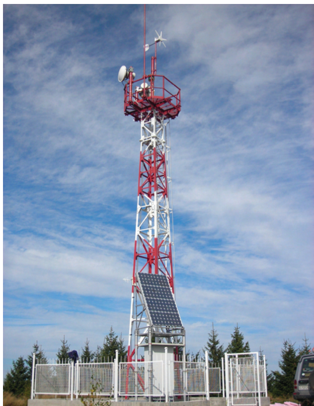
Fig 5 Photo of the realized alternative hybrid energy supply for TELEKOM Serbia microwave communication node at hard to reach Orlovac mountain location in south east part of Serbia (1670m Above Sea Level)
