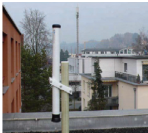
Fig. 8. Sensor located outdoor on the roof.
