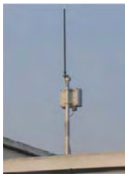
Figure 2c. LR outdoor installation
