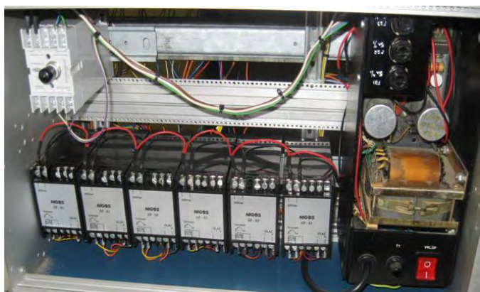
Fig. 3. Temperature and vibration transmitters mounted in a rack
