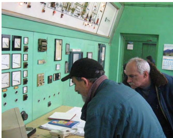
Fig. 4. Control room in the sulfuric acid plant
