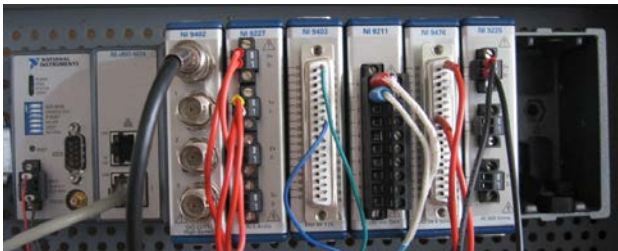
Fig. 2. cRIO controller with modules
