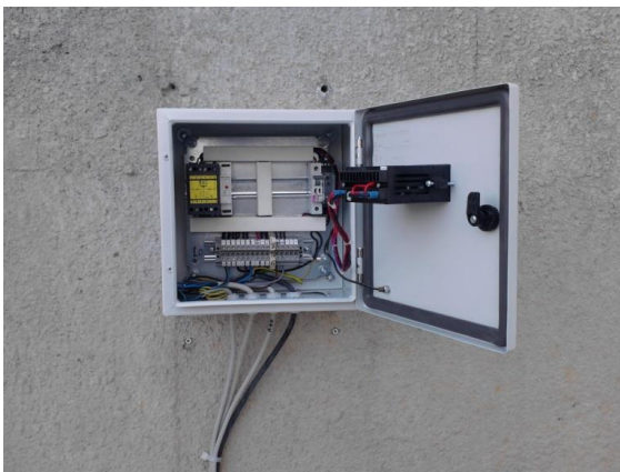
Fig. 7. The cabinet with elements of the electric motor overloads protection system
